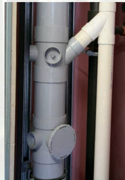
Secondary ventilated stack
