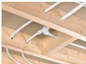
Easy cabling. Fewer joints
