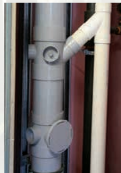
Secondary ventilated stack
