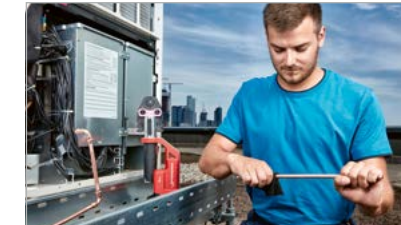
4. Clean the tube end with a circular movement, avoiding grooves that run parallel to the tube.
