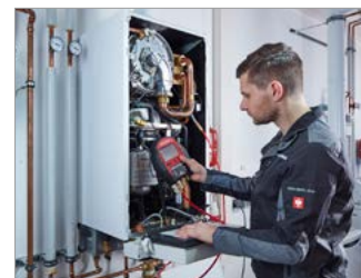
Testing of gas pressure regulators
