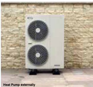
Heat Pump externally
