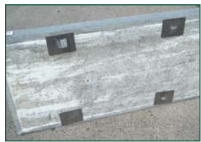
3. Insert all 4 base plates through the light weight slab and reposition to the required location of the ASHP unit.
