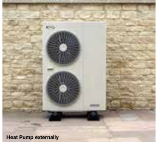
Heat Pump externally
