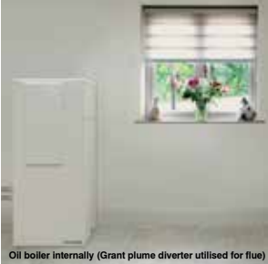
Oil boiler internally (Grant plume diverter utilised for flue)
