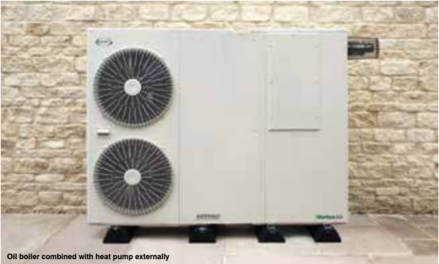
Oil boiler combined with heat pump externally
