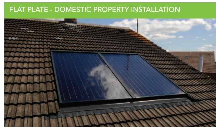
Domestic property with a Vokera Zenith Inset installation
