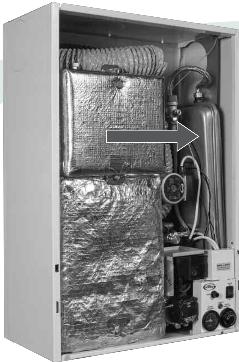
Figure 7-3: Expansion Vessel location
