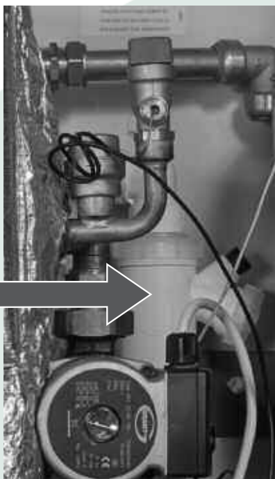
Figure 6-2: Condensate trap location in-situ
