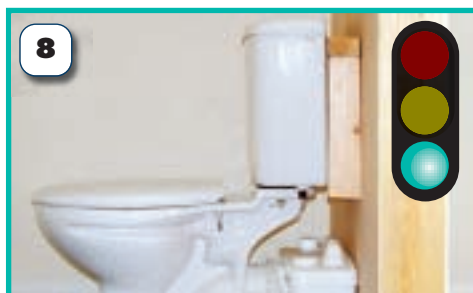
11 Since many close coupled WC suites do not have the space between the WC pan spigot and the wall, you may have to batten the cistern off the wall to make room for the Saniflo. However Sanislim will fit behind most closed coupled WC suites without the need for this.
