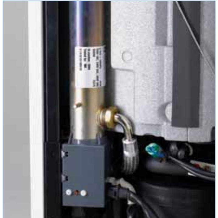
Additional electrical heater in three steps 3/6/9kW that is controlled automatically by control unit
