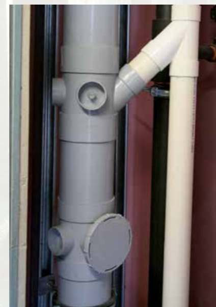
Secondary ventilated stack
